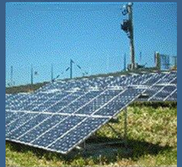
Solar Power Station
